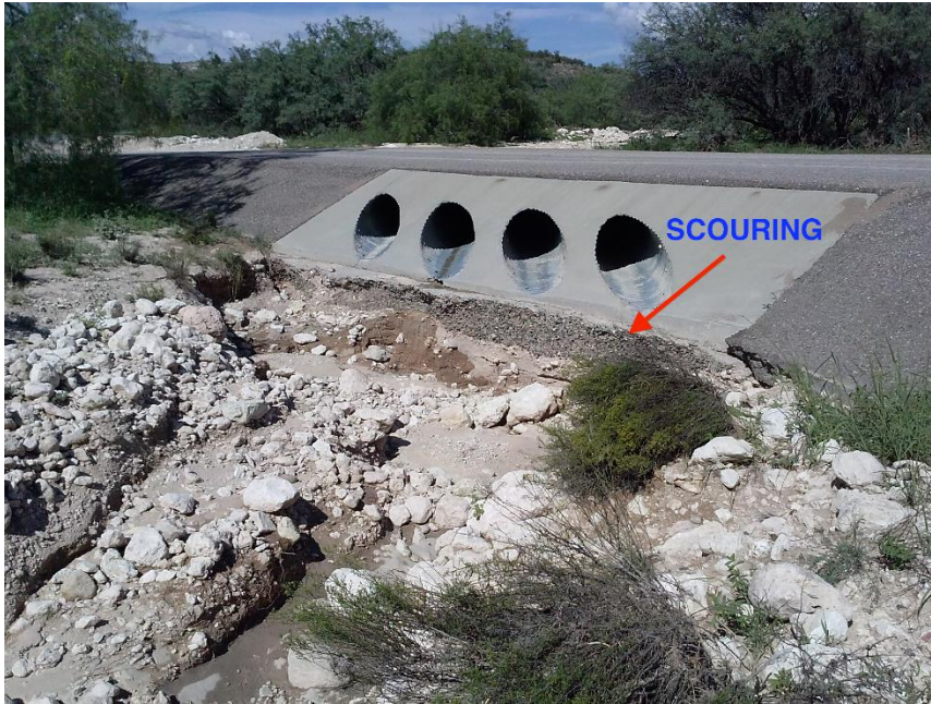
Figure 5.4: Pipes Exit with some scour forming
